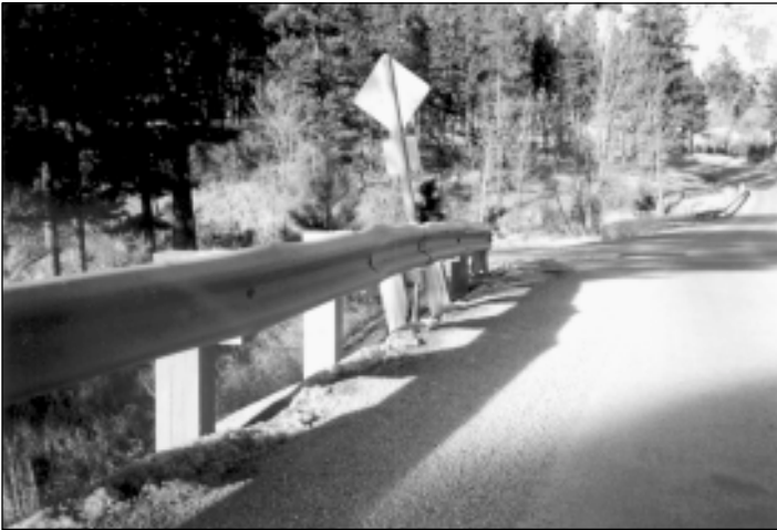
The support posts of this guardrail may be broken.
